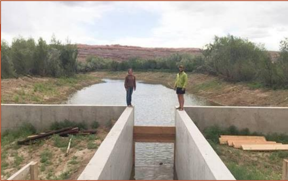
Two members of the monitoring team stand on a stop-log “gate” system that slows the water moving between the river and the wetland pond
